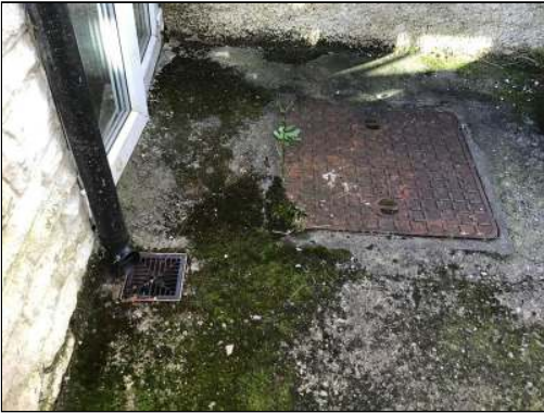
Photo - 70 Manhole in rear garden
