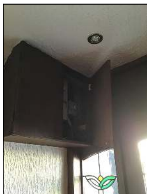
Photo - 46 Fuse board door is loose.
