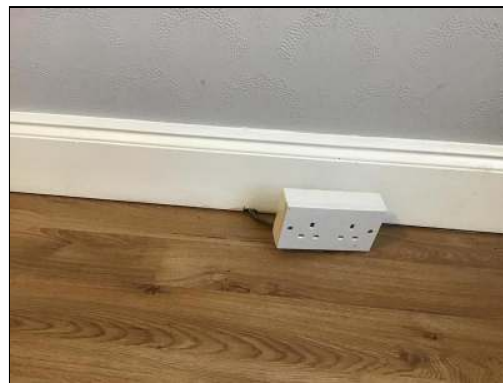
Photo - 61 Sockets too close to the floor, and loose wiring.
