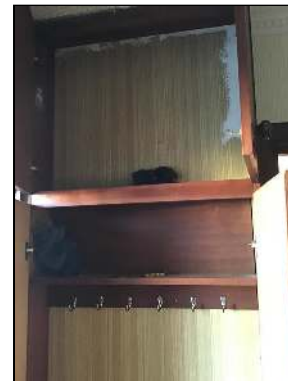
Photo - 45 Built in unit in hall.
