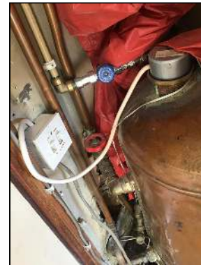
Photo - 68 No labels on valves and stopcocks in the hotpress
