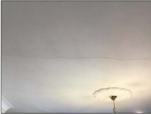
Photo - 29 Shrinkage cracks to be investigated and repaired.
