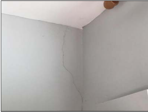
Photo - 35 Shrinkage crack in rear bedroom to be investigated and repaired.
