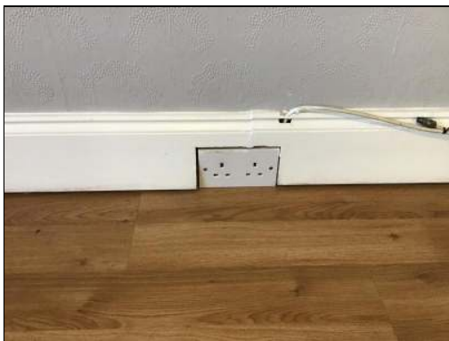
Photo - 60 Sockets too close to the floor
