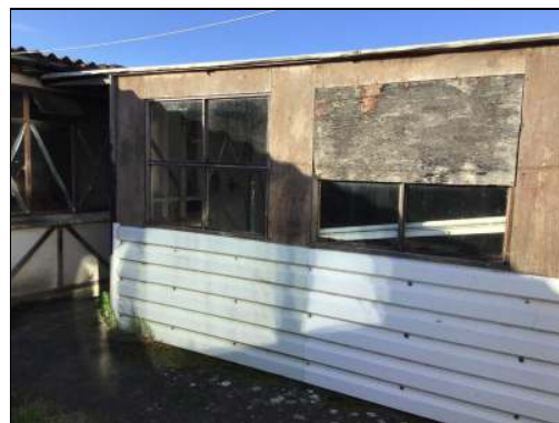
Photo - 76 Workshop structure in poor condition. Roof is sagging and leaking.
