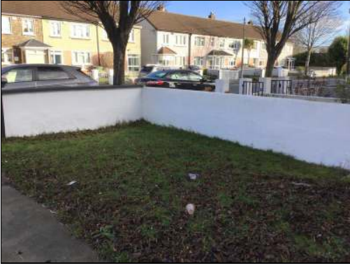
Photo - 84 Front boundary wall
