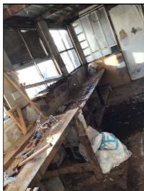
Photo - 75 Workshop structure in poor condition. Roof is sagging and leaking.
