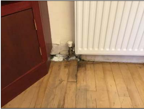
Photo - 66 Poor workmanship at heating pipes.
