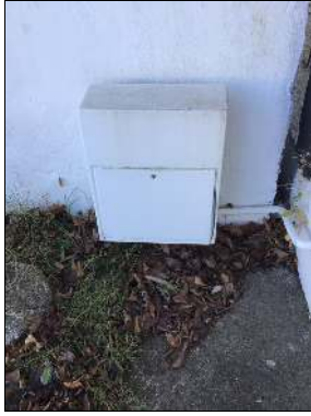
Photo - 62 Gas meter box in front garden
