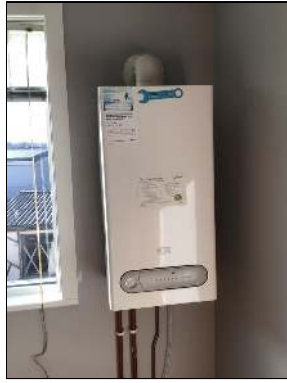
Photo - 64 Boiler to be serviced.
