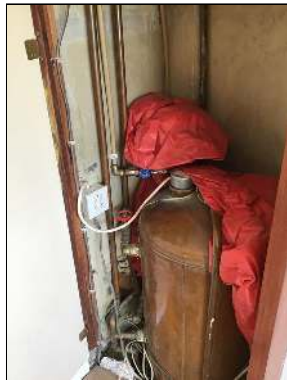
Photo - 67 Cylinder not adequately insulated.
