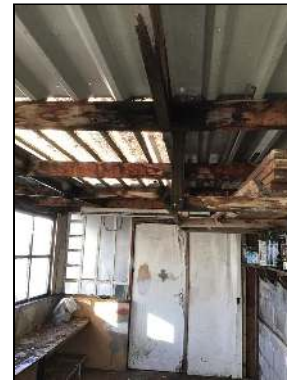
Photo - 74 Workshop structure in poor condition. Roof is sagging and leaking.
