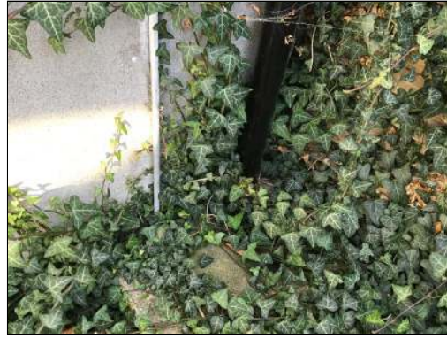
Photo - 5 Gully trap to rear is overgrown.
