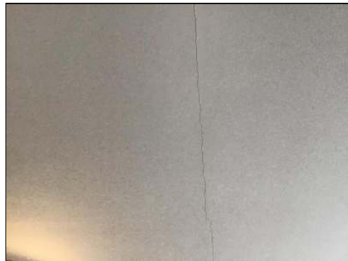
Photo - 32 Shrinkage cracks in ceilings to be monitored for possible future deterioration.
