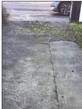
Photo - 73 The private gardens are in need of attention. Driveway is cracked.
