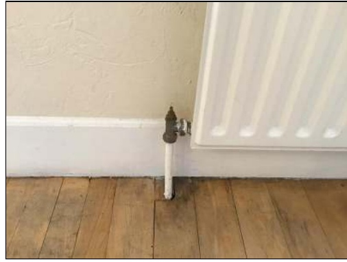
Photo - 65 Radiator caps missing.
