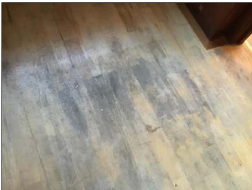
Photo - 36 Laminate finish. Badly stained in some areas.
