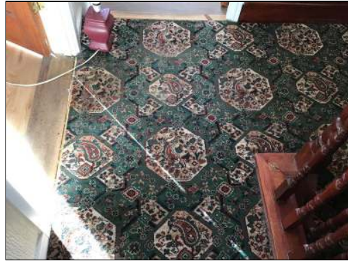
Photo - 39 Carpet on stairs and landing. Very creaky floor on landing.
