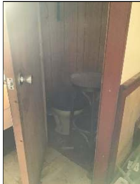
Photo - 81 Sub standard WC fitted in Shed, not connected
