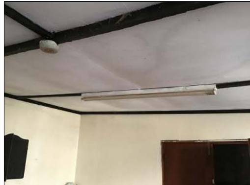
Photo - 82 Shed roof is sagging
