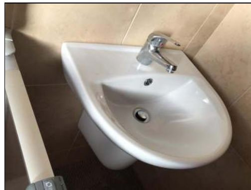
Photo - 53 Wash hand basin
