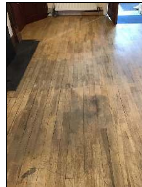
Photo - 37 Laminate finish. Badly stained in some areas.
