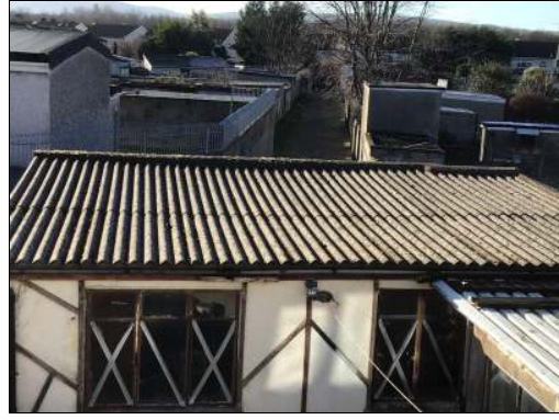
Photo - 78 Asbestos sheeting on shed roof
