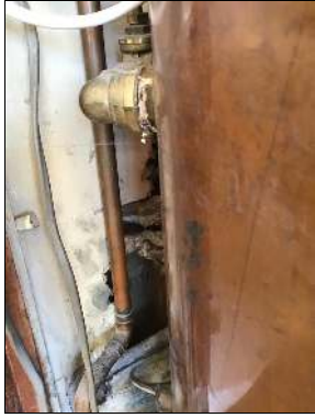
Photo - 69 No labels on valves and stopcocks in the hotpress
