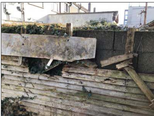
Photo - 19 Fence in very poor condition
