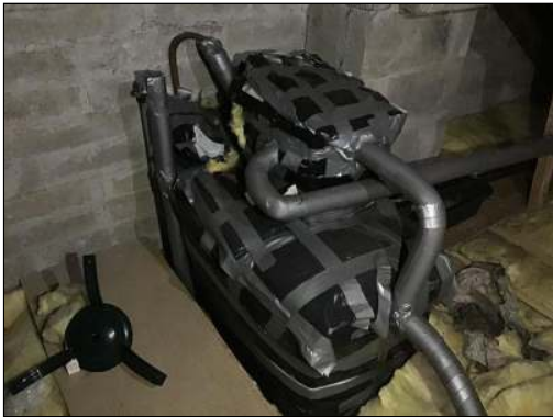
Photo - 55 Fully insulated tank and pipes in attic
